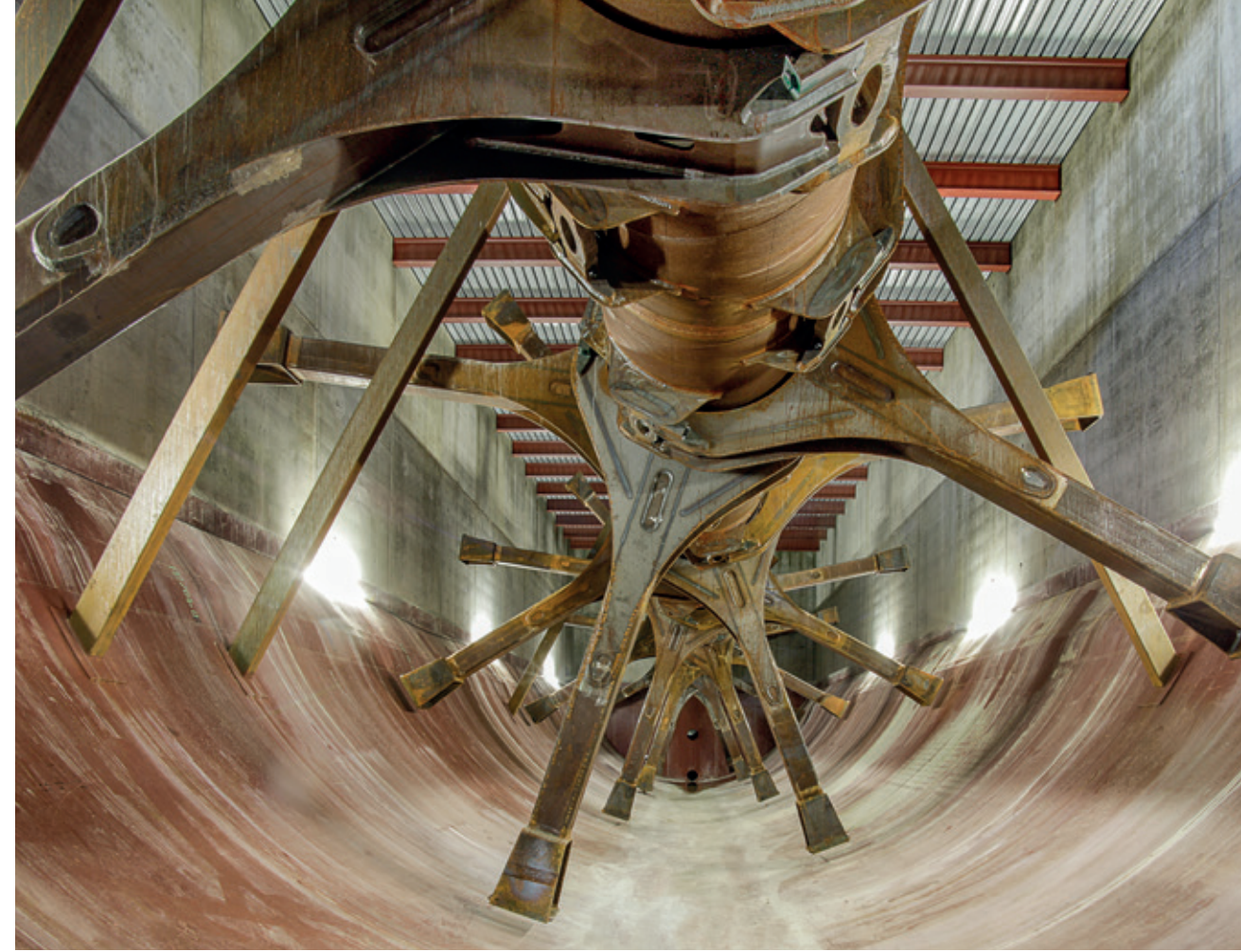
TTV digester - internal view
