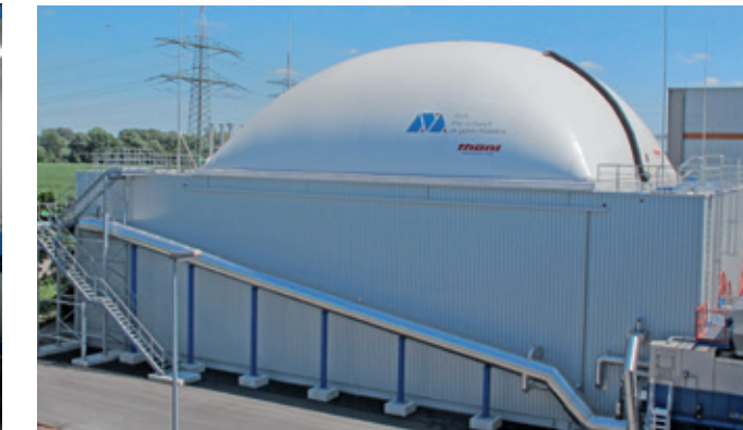
Biogas plant with gas storage unit
